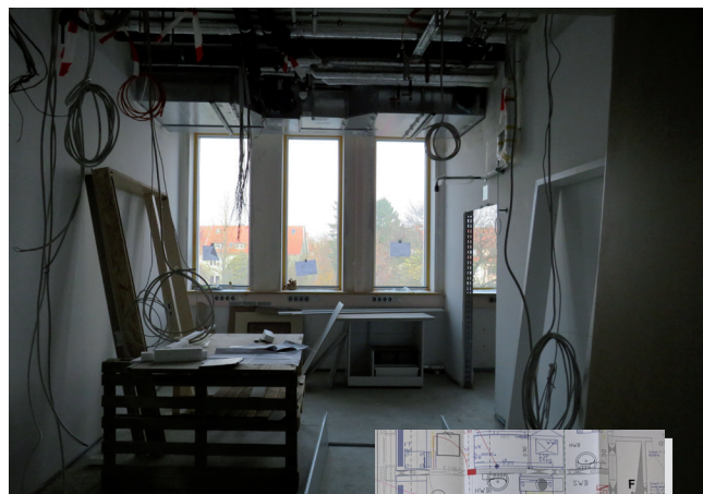
Figure 8: The new S2 biosafety laboratory under construction in the new Chemistry extension building.
